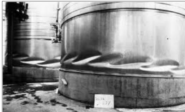
Figure 1: Shell structures damages due to earthquake
