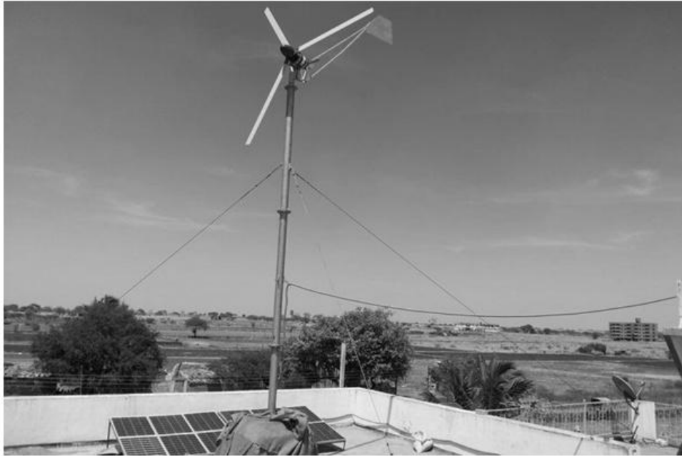
Figure 2: Wind Turbine on Roof Top [15]
