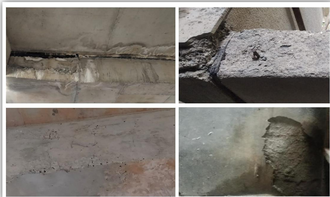
Figure 2: Freeze Thaw Observed in the Building Constructed with Normal Concrete
