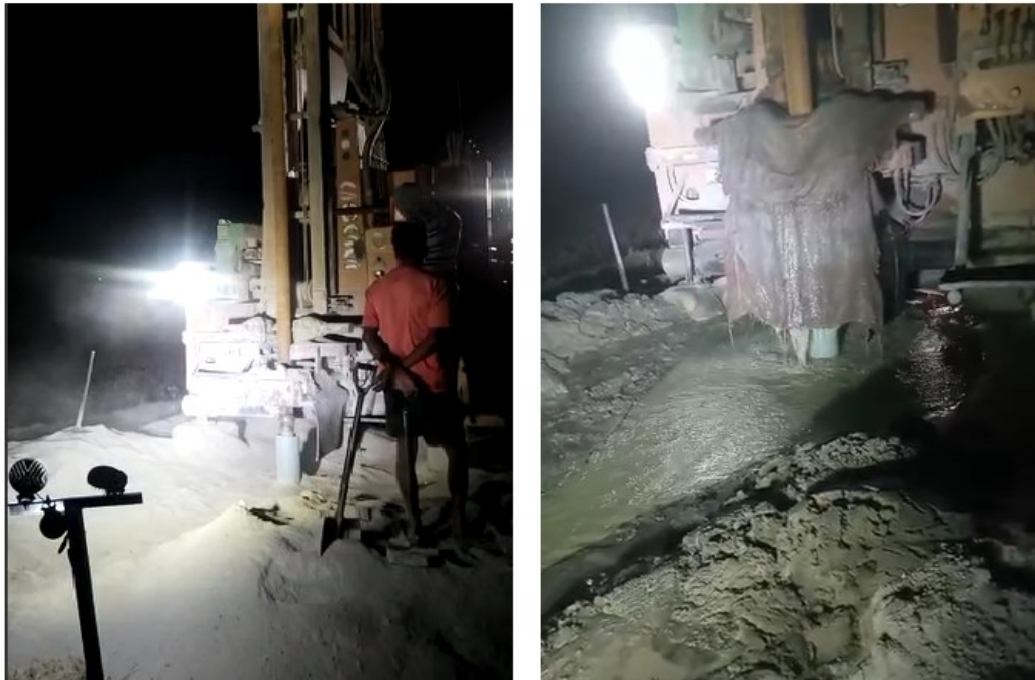
Figure 3: Bore hole drilled in Koviloothu village farm showing Charnockite hard rock formation grinded as powder and deeper aquifer consisting water at deeper depth.
