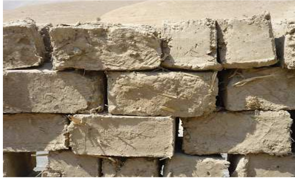
Figure 8: Stabilized Mud Blocks
