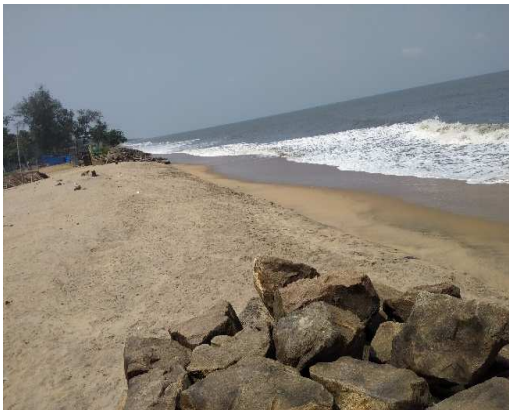
Figure 11: Seawalls with Gaps
