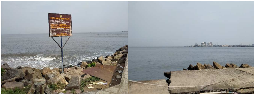
Figure 5: Warning board at Fort Kochi Figure 6: Damaged pathways at Fort Kochi
