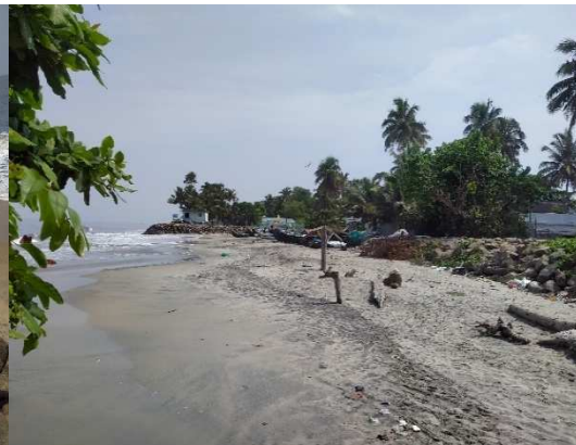
Figure 12: Seawall gap at Beach Road
