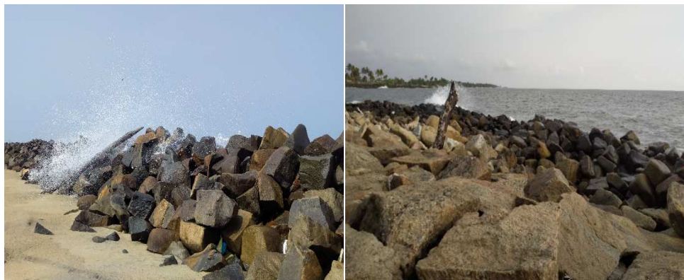
Figure 7: Collapsed Seawall Figure 8: New Layers of Rocks Replaced old ones
