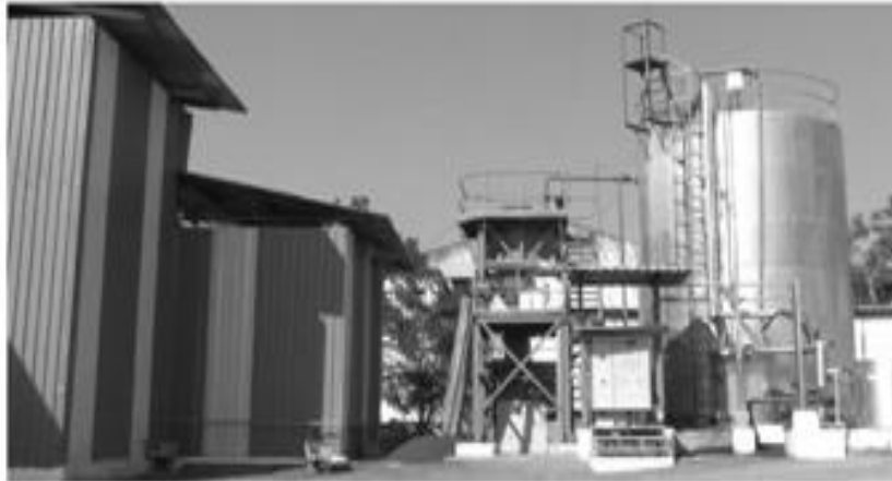
Bioreactor/ Digester at Bio-CNG Production Centre
