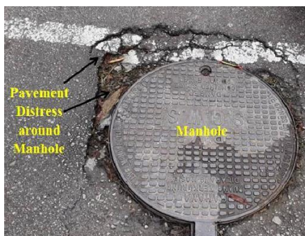
(i) Distress occurred around manhole built in flexible pavement.
