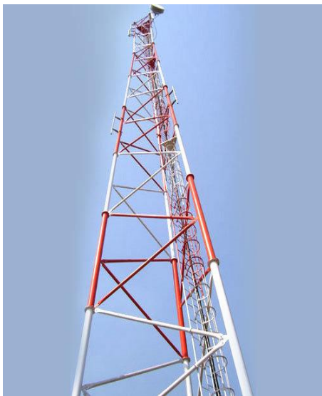
Figure 7: Fabricated Steel Tower
