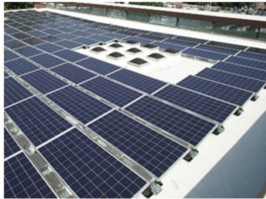
Figure 2: Photo Voltaic Panels. Source: [42]
