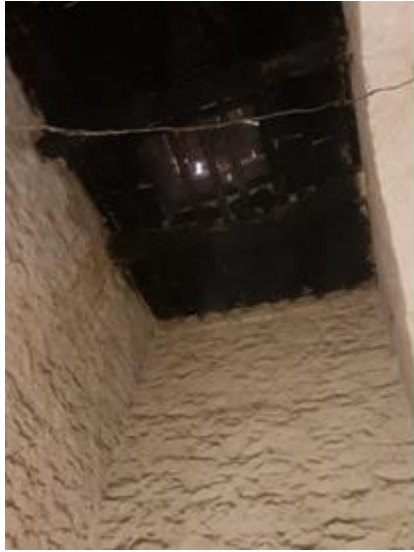
Fig: 22(author) Roof ventilator which can be opened or closed when required. Even seasonal wise, in rainy it can be closed.
