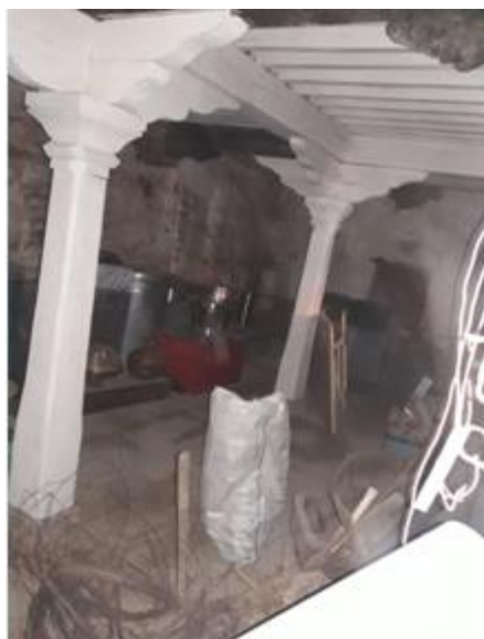
Fig: 16 (author) store room - wooden columns supporting the beams .mud roof covered with wooden planks.
