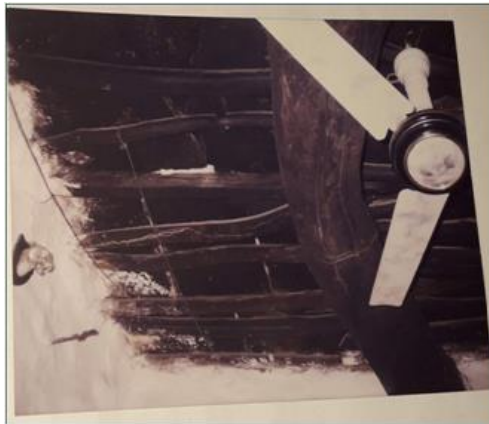
Fig: 10(author) Dhabhi- wooden beams, rafters, planks above that mud moulds are placed with proper ramming with wooden mallet.
