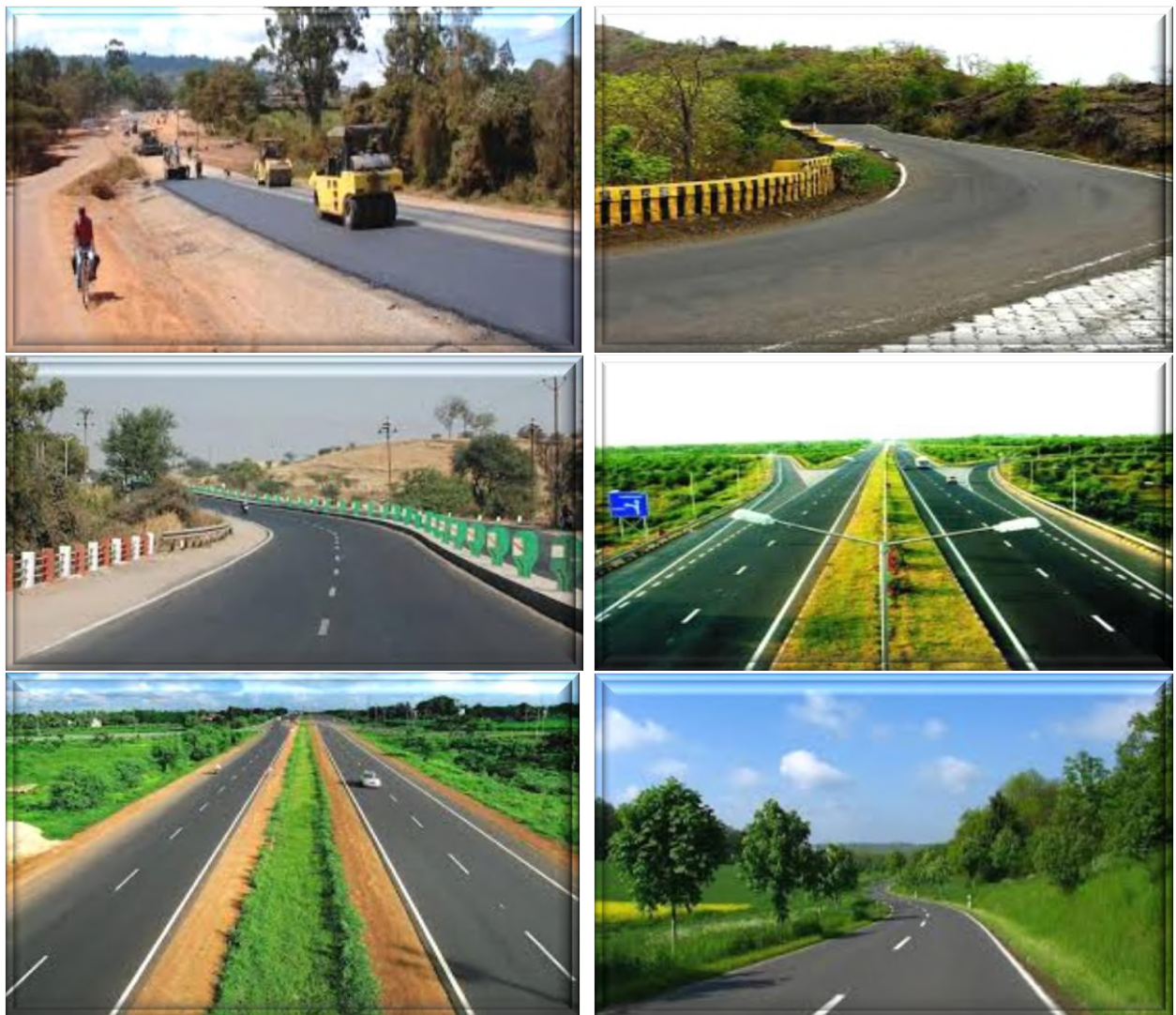
Figure 13 (a): Mitigation Enhancement as per Alignment Design Phase to Reduce Tree Cutting and Compensatory Plantation Relevance.
