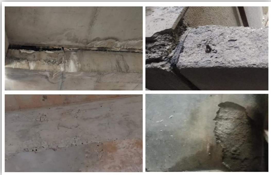
Figure 2: Freeze thaw observed in the building constructed with normal concrete
