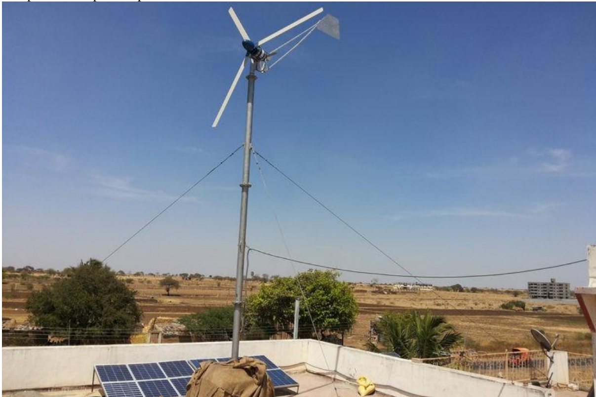
Figure 2. Wind turbine on roof top
