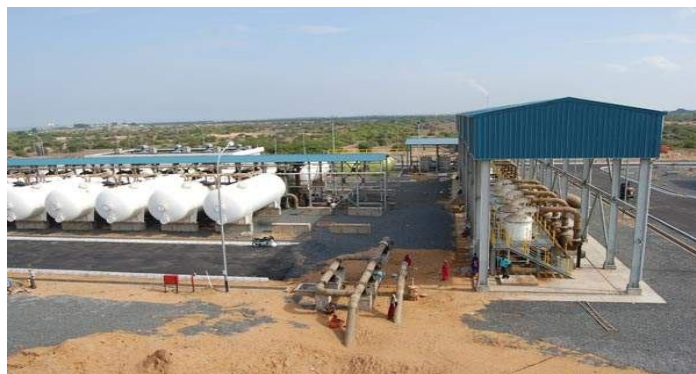
Fig.4: The Minjur Desalination Plant (Tamil Nadu- Chennai, India)
