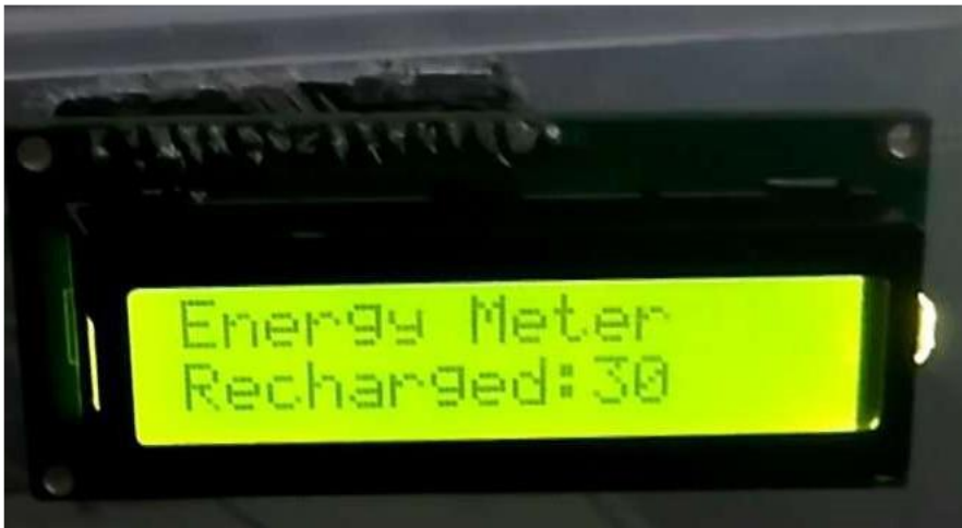
Figure.16 Energy meter Recharged by 30 rupees.
