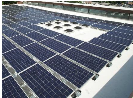
Figure 2: Photo Voltaic Panels. Source: [42]
