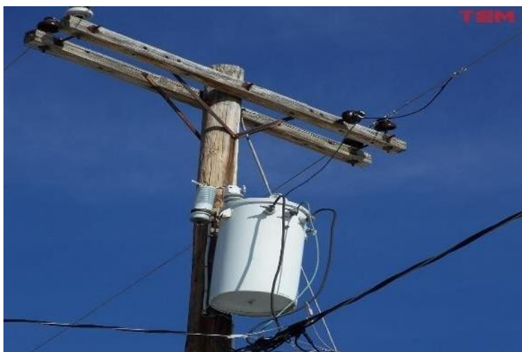
Figure 2. Pole-mounted distribution transformer
